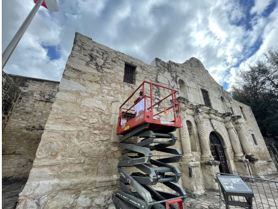
The pigment extraction will require a electric scissor lift on the plaza-facing part of the Church.
