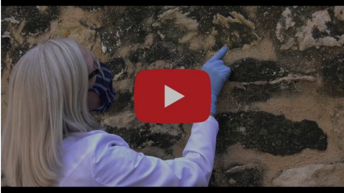
Alamo Conservator Pamela Rosser details the Long Barrack repairs and cleaning process.
